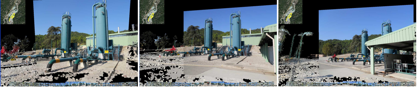
Figure 2: Live navigation screenshots using the 3DNSITE viewer. Interactive 3D navigation over the gas storage site of Geomethane in Manosque (France). This site has been used as training emergency scenario on the framework involving 3DNSITE (the 3DNSITE system is in charge to store, stream(server side) and visualize(client side) tridimensional hybrid data) involving the Operational Center of the Fire and Rescue Services of Alpes de Hautes, the local Gendarmerie and many real crisis managers and first responders. The company is an underground hydrocarbon storage site with a 7.5 million m3 storage capacity. It was created in 1969 and is classified as a SEVESO (high-risk production site). Due to this classification has been an excellent test case for the all system.
