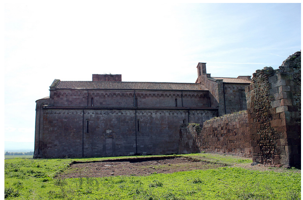
Figure 4. Area 5100: in the background, southwards, the west wall of the cathedral. Right: the perimeter wall of the bishop citadel.
