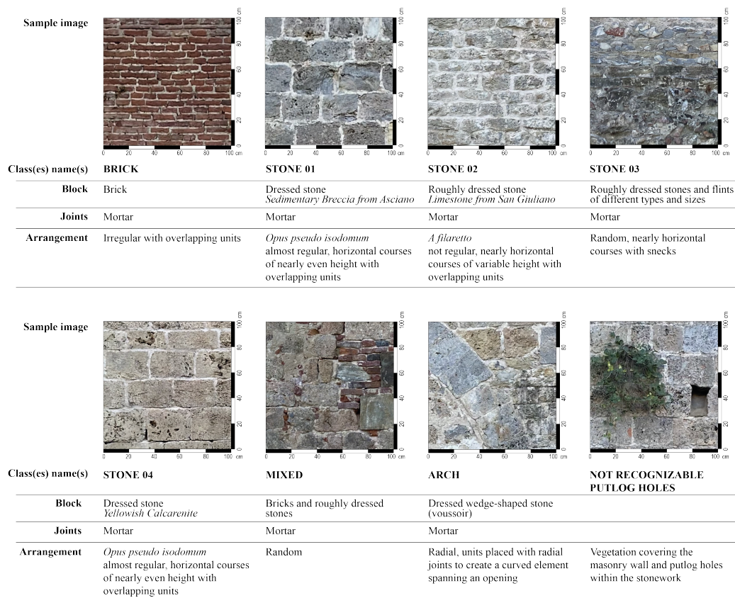
Fig. 2. Semantic classes of the city walls of Pisa. Not recognizable objects and putlog holes (bottom-right) are two separate classes.
