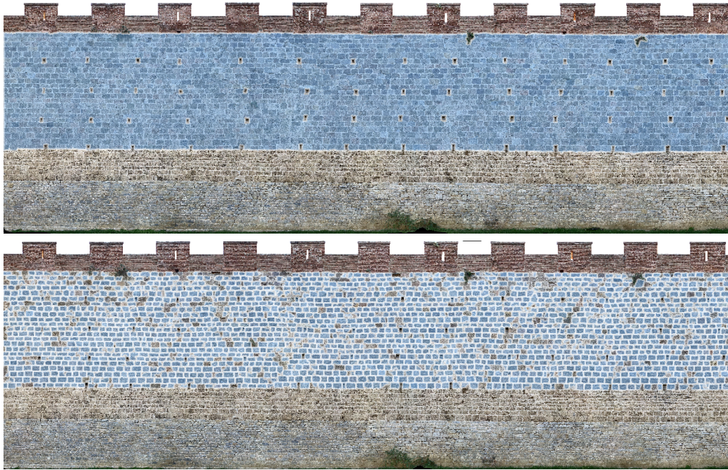
Fig. 12. The semantic class STONE 01 covers 176 square meters in the Vittorio Veneto D map (Top). The bricks segmentation tool traced 1839 stones for this area (Bottom). Most of the stones are correctly marked; the missing or partially-traced bricks can later be fixed by using the positive/negative clicks tool.
